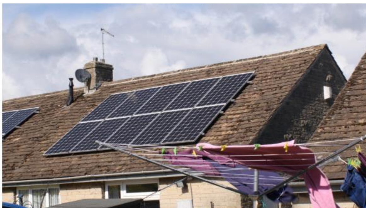
Figure 23: Solar PV Installation in Barnsley
