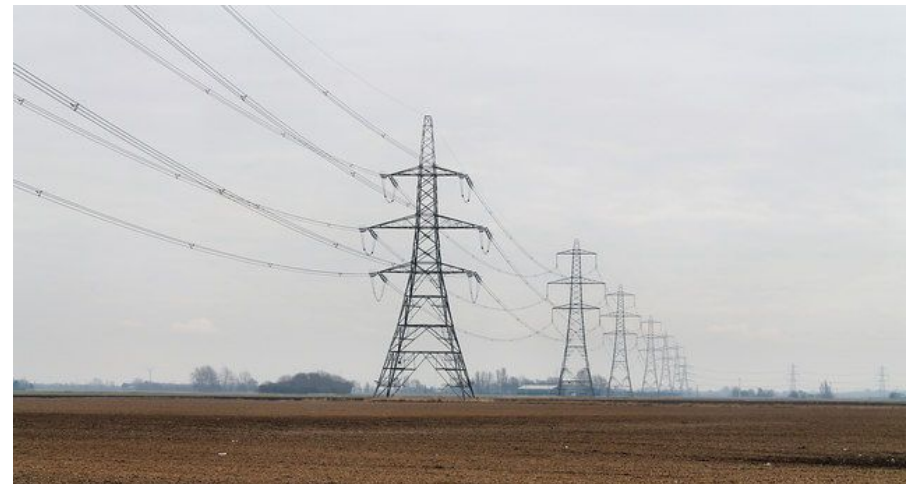
The electrical infrastructure will have to be reinforced to support increased demand and a more distributed supply with more renewable energy
